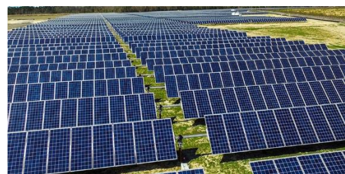
20200 Solar Panels 13.5MWp
